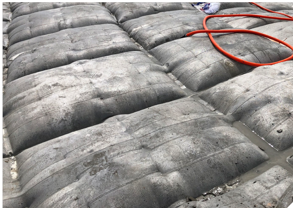
Articulating Block showing separation between blocks
